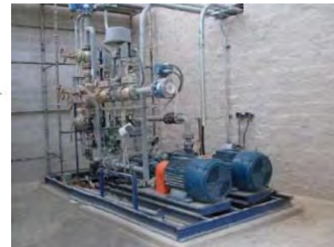
High Pressure Pumps
