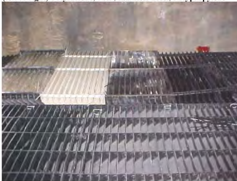
Figure 2. Test Installation at APS's Cholla Station, Unit 2: Materials (left to right) Polysulfone, FRP, Stainless Steel, Polypropylene
