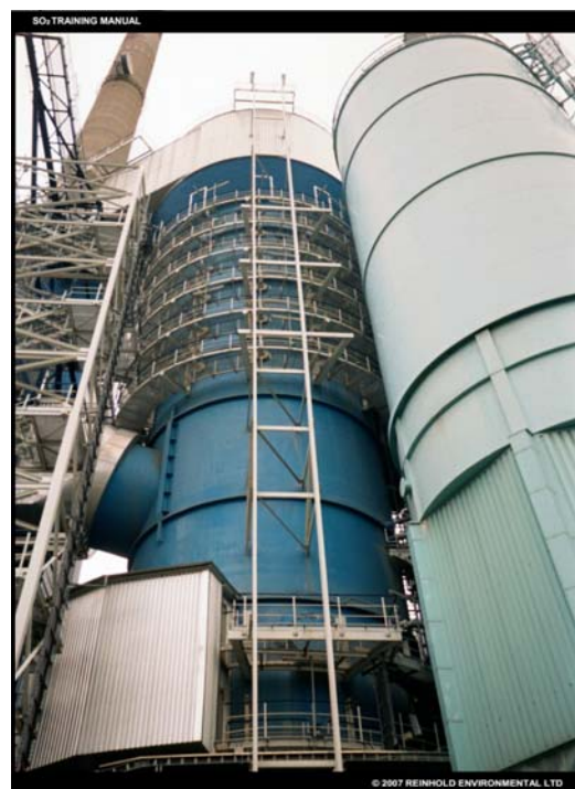
Wet Limestone Scrubber at a German Power Plant Used with permission
