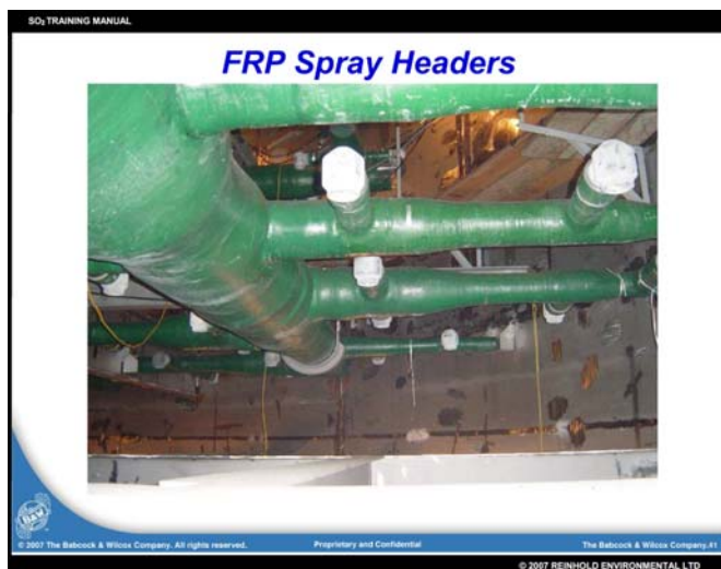
Spray Headers - FRP
