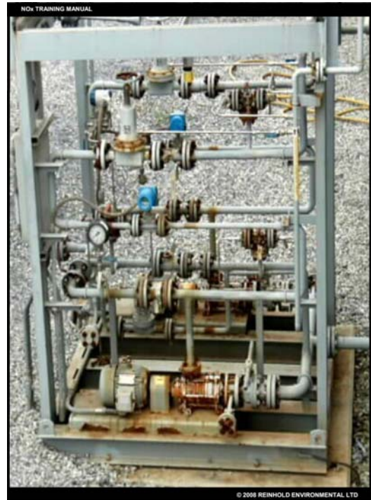
Liquid Ammonia Forwarding Pump Skid (Used with permission)
