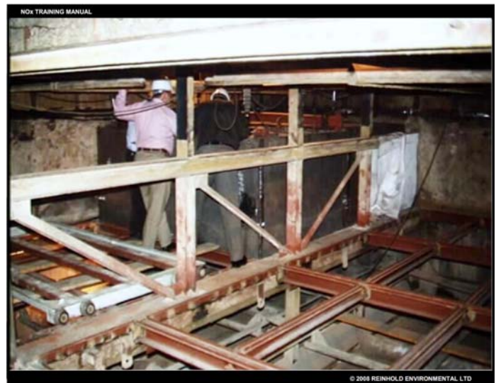
Catalyst Supports and Transfer Cart (Used with permission)
