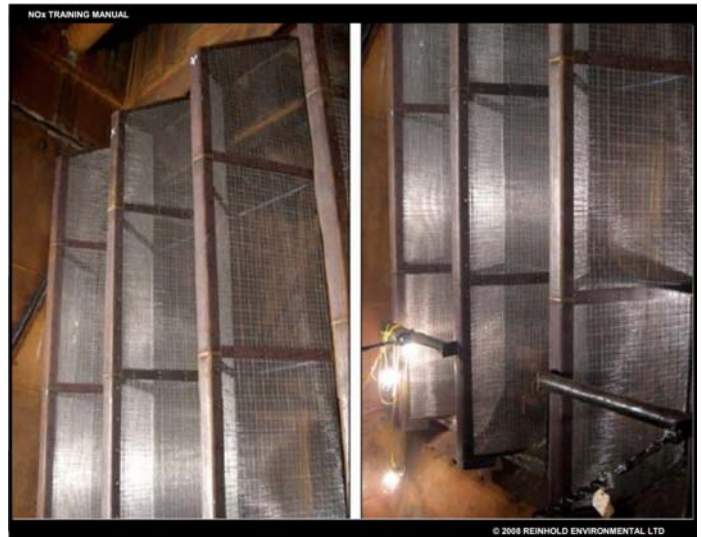
LPA Screens (Courtesy of Evonik Energy Services)
