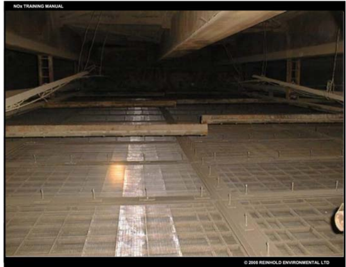
Rake Type Soot Blower (Used with permission)
