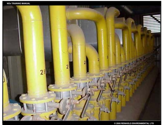
Ammonia Injection Piping (Used with permission)
