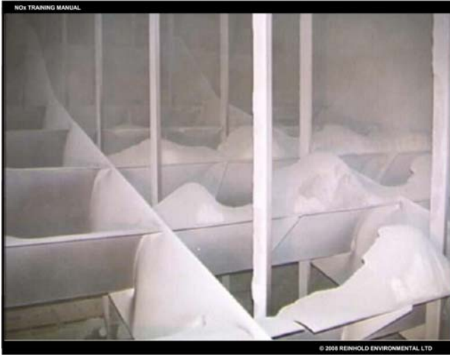
Turning Vane Deposits - 1 (Used with permission)
