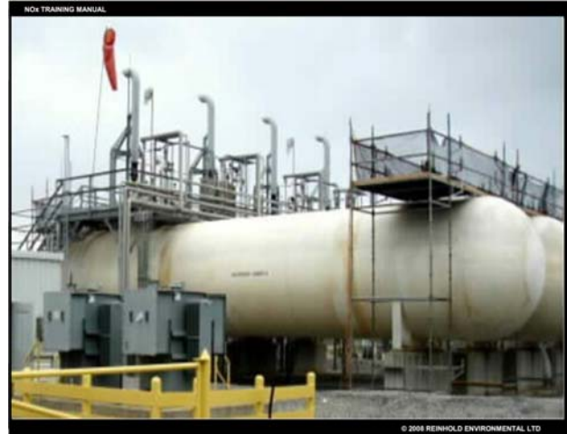
Ammonia Storage Area (Used with permission)
