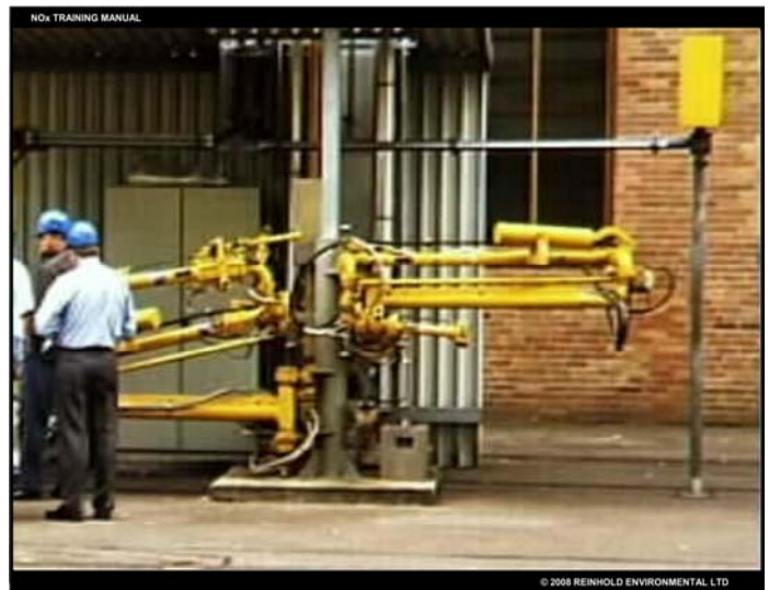
Ammonia Unloading Station (Used with permission)
