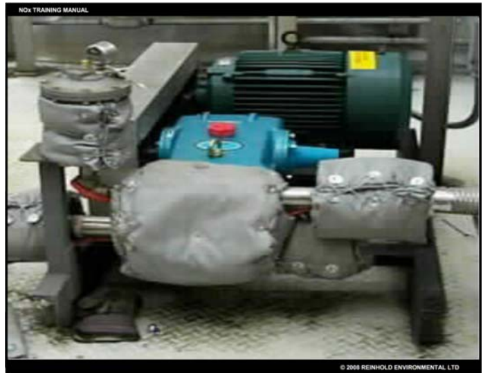
Urea Hydrolyzer Feed Pump (Used with permission)
