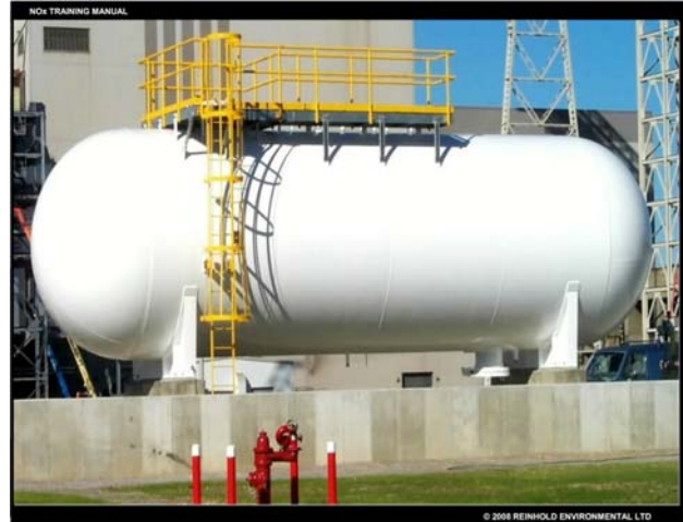
Ammonia Storage Vessel (Used with permission)
