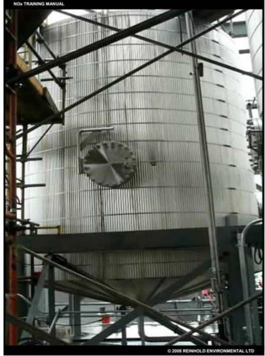
Urea Small Solution Storage Tank (Used with permission)
