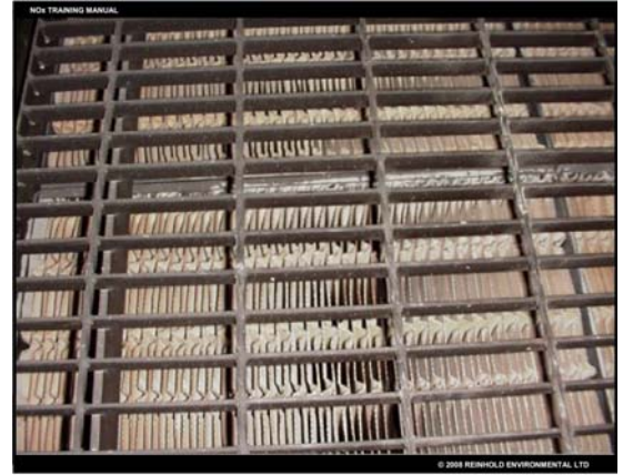
As-Installed Plate Catalyst with Grating (Used with permission)
