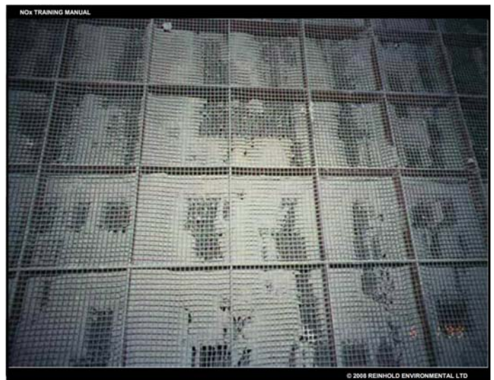
Economizer Leak Aftermath (Used with permission)
