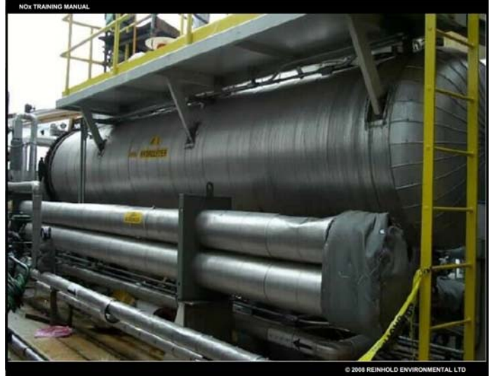
Urea Hydrolyzer (Used with permission)
