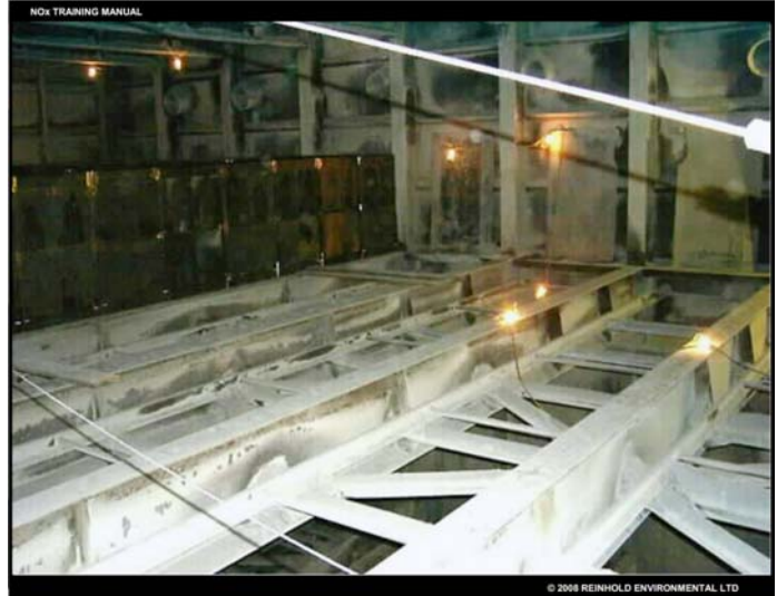
Catalyst Support Beams (Used with permission)
