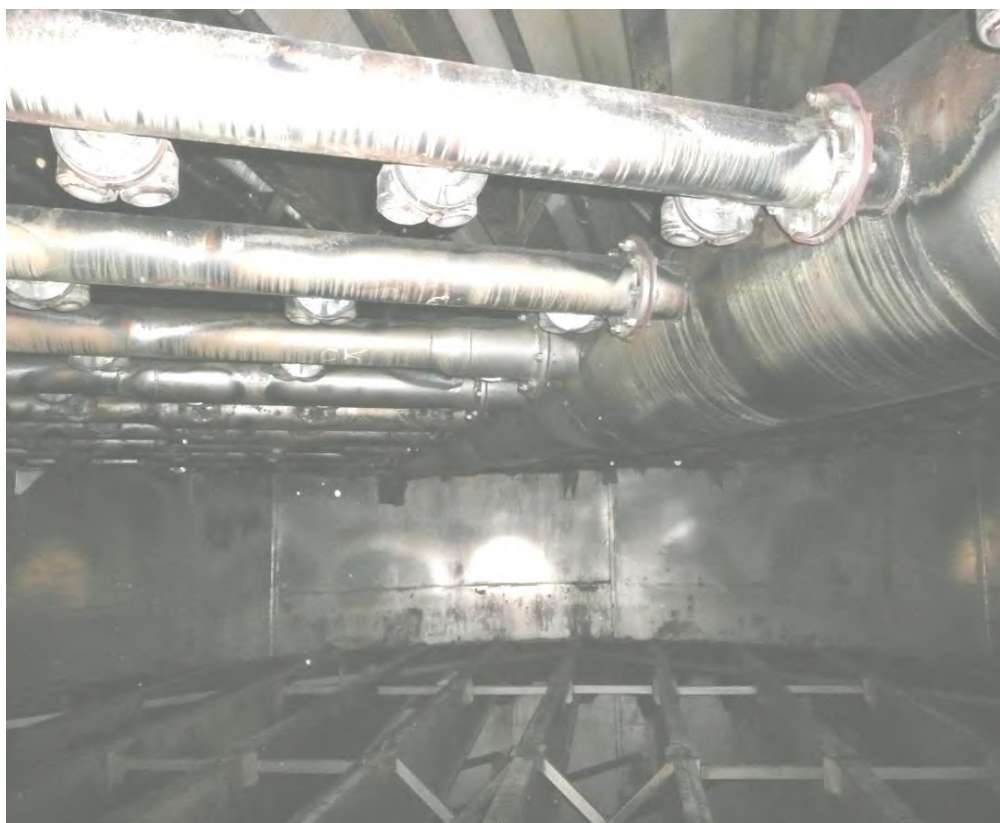
Nozzles Above WFC
