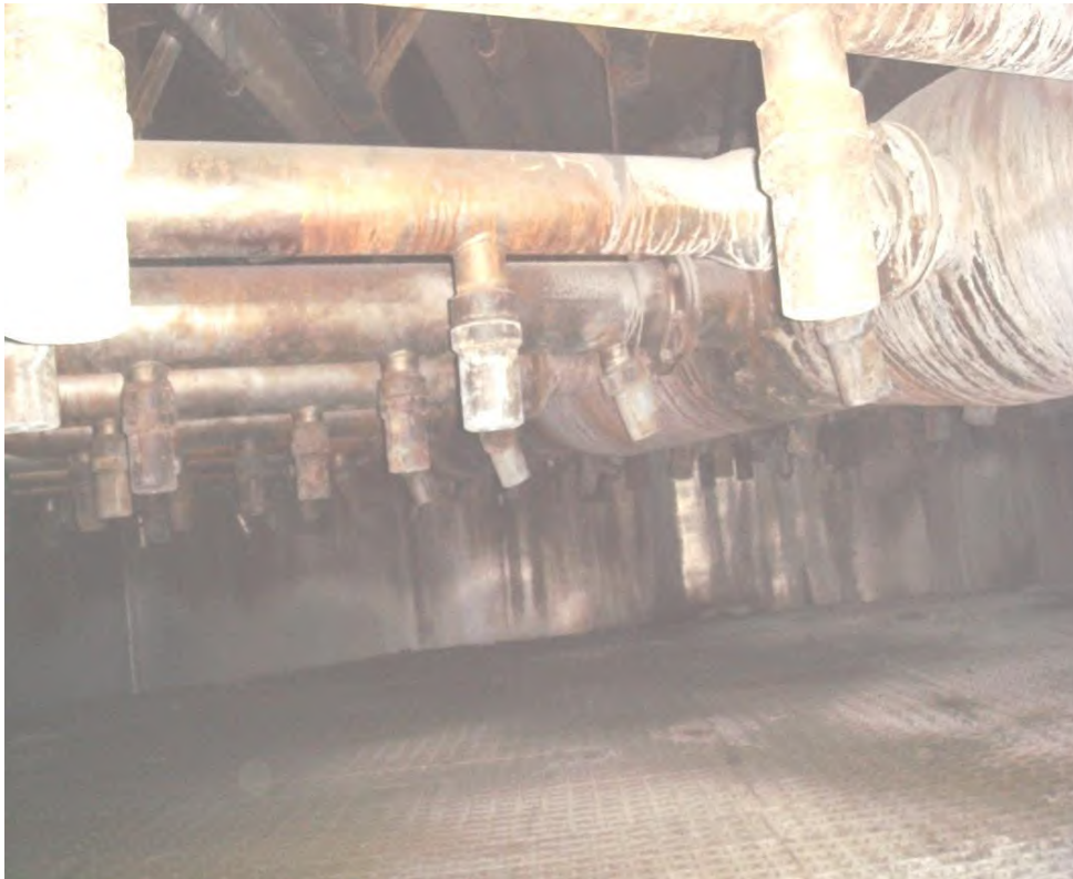
Nozzles Above WFC
