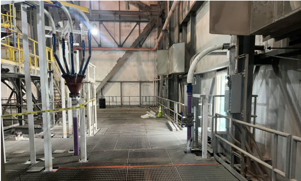
Vertical flow to splitter for even splitting.
