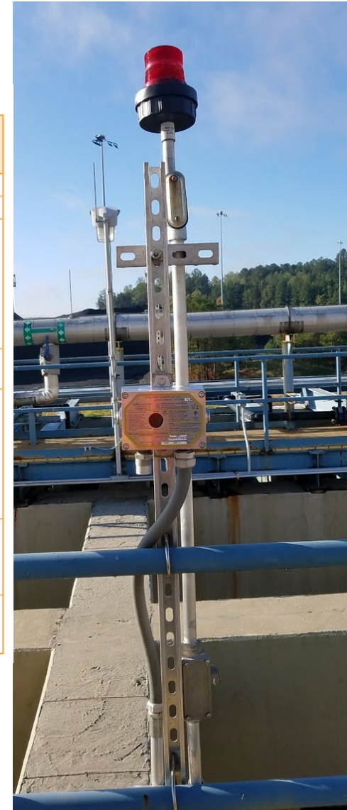
Bioreactor - H 2 S Monitor
